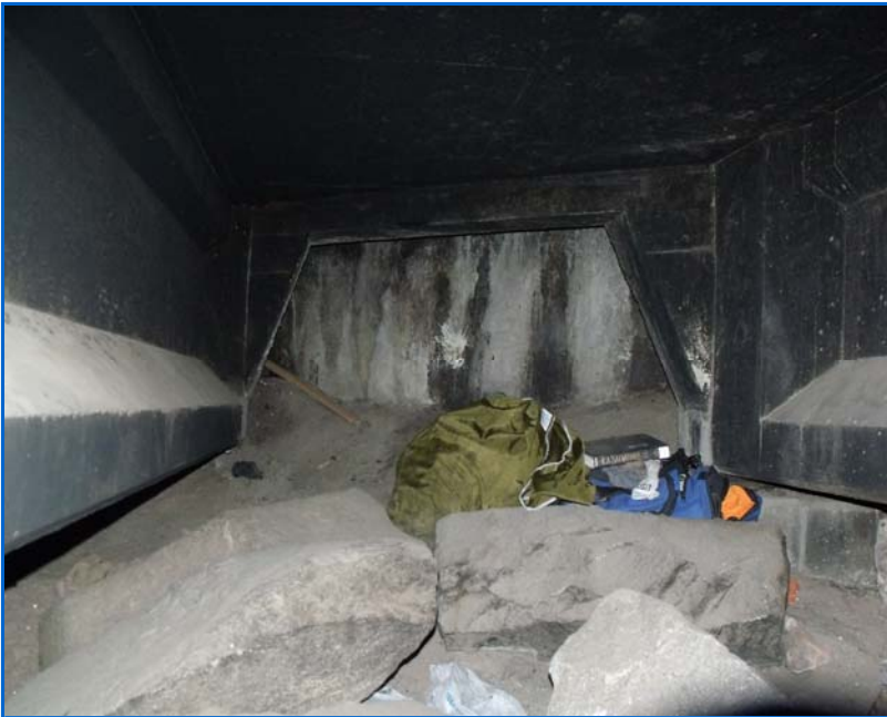
I17DE Piles of sand and debris along abutment seats due to failed and opened jts above.JPG
