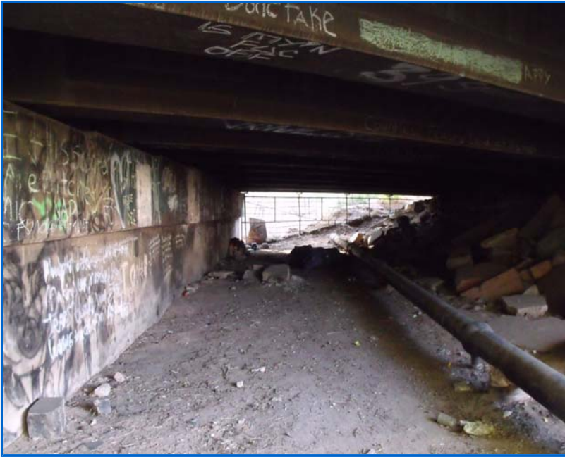
I17DE Span 1 with rampant graffiti and soot due to homeless occupying closed off spans.JPG
